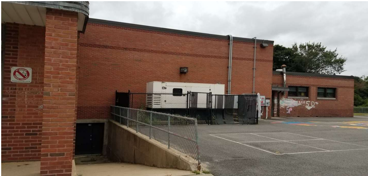
This generator is beyond its useful life, and no longer code compliant. The exhaust stack needs to be well above the building, or the generator needs to be much further away. This is now required to prevent exhaust fumes from entering the building.
