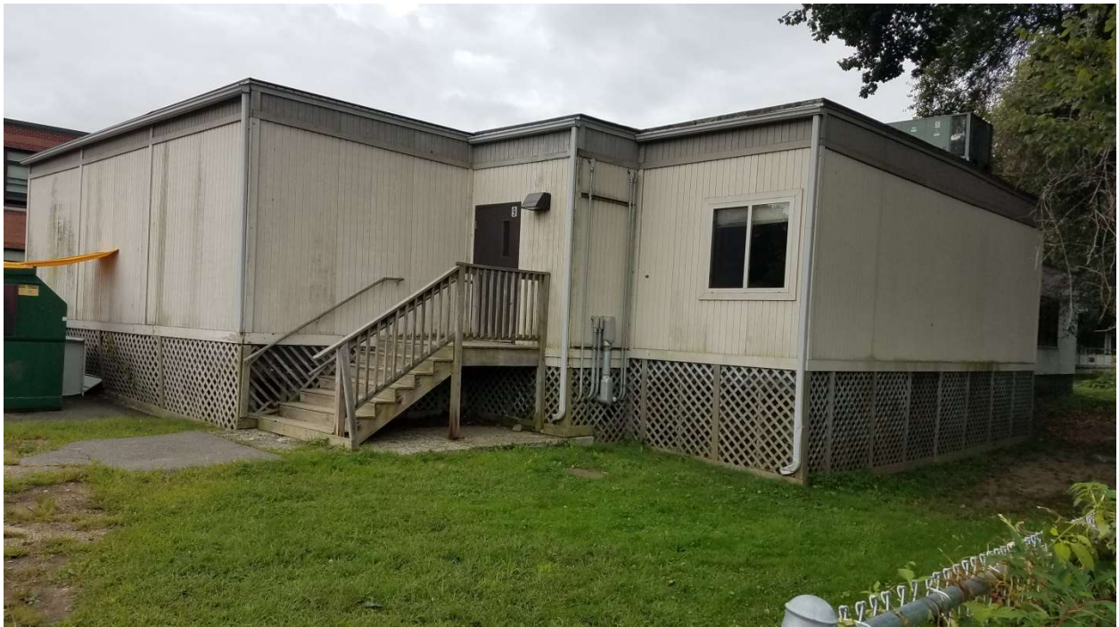
Most of the modulares sit on jacks or cinder blocks. The foundations are then covered with lattice. This means that the floors are exposed to the elements.
