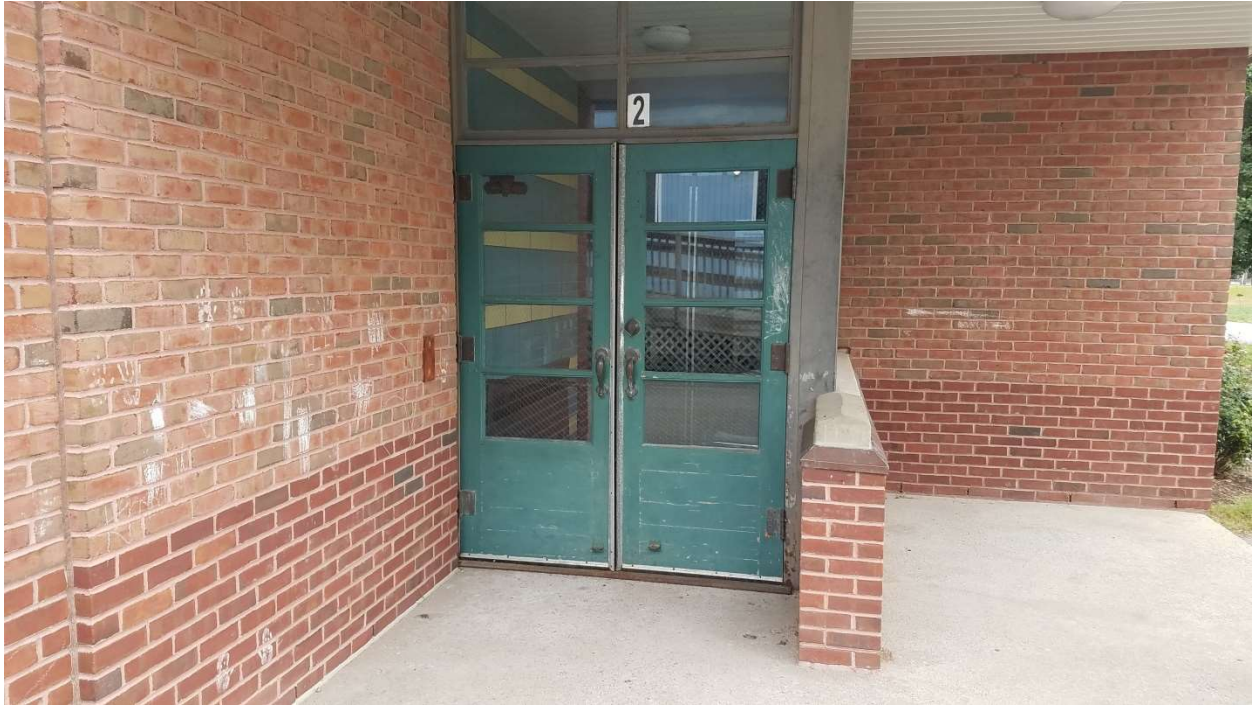
Some doors are not only inaccessible, but original to the building and in very poor condition.
