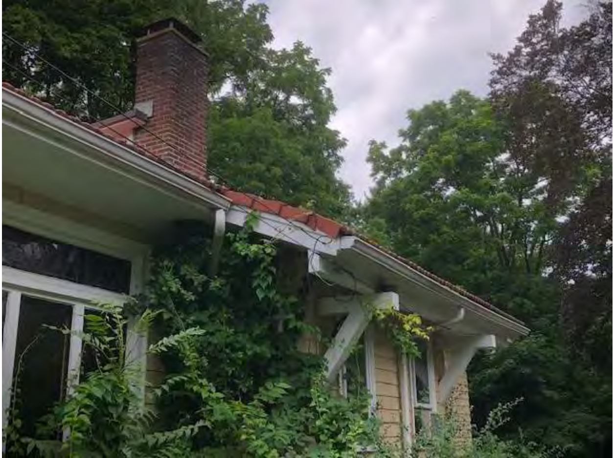
145 Warren Street, view looking northwest of east side, tile roof and struts
