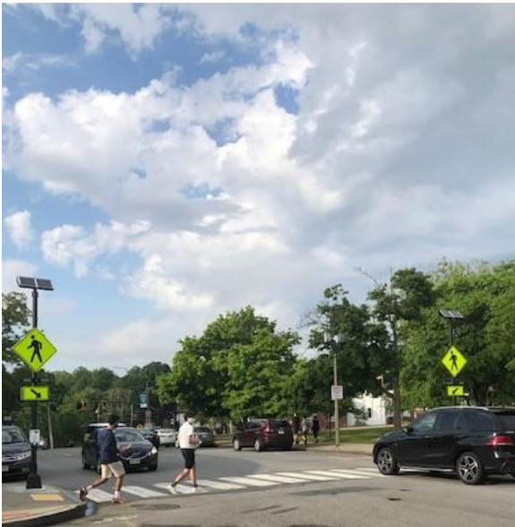
Rectangular Rapid Flashing Beacons at Newton Center
