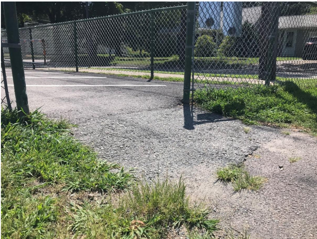
Above: Existing conditions including a sloped asphalt patch as individuals leave the parking lot.
