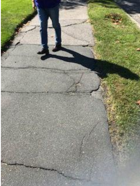
5. Repair unsafe sidewalks around park.
