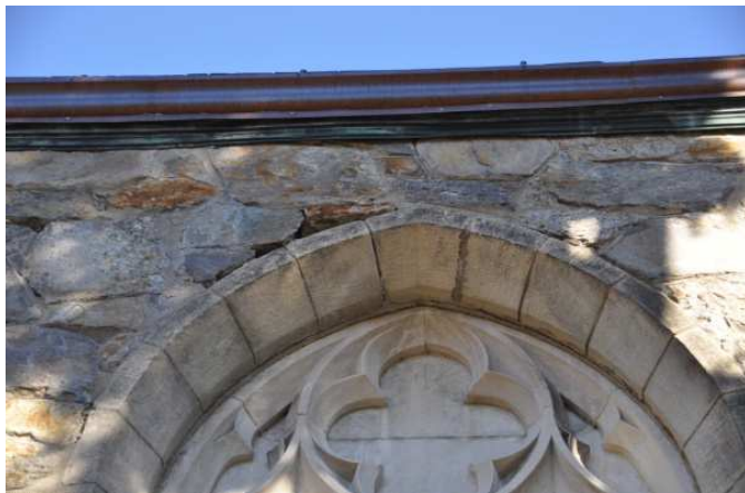
Photo 4: Mortar Deterioration at Blank Window
