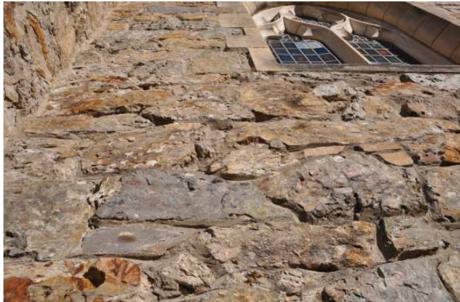
Photo 3: Mortar Deterioration on Church
