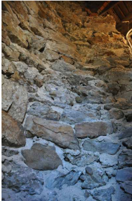
Photo 13: Mortar Deterioration inside tower
