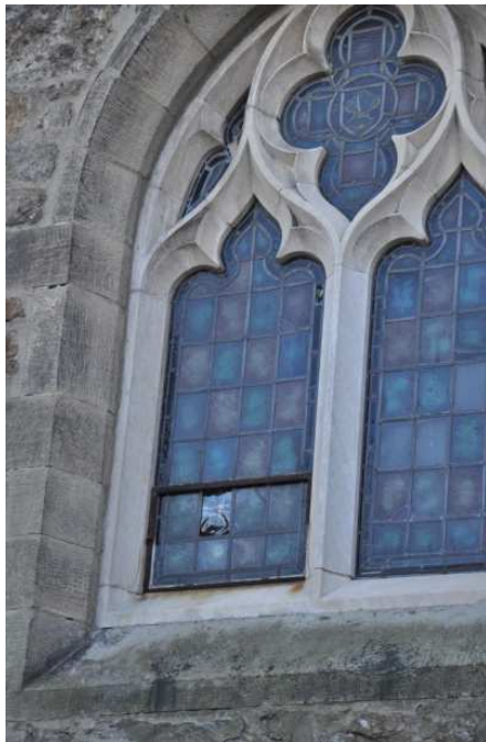
Photo 12: Broken Pane in Nave Window
