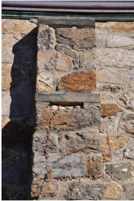
Photo 5: Mortar Deterioration at Coping Stone
