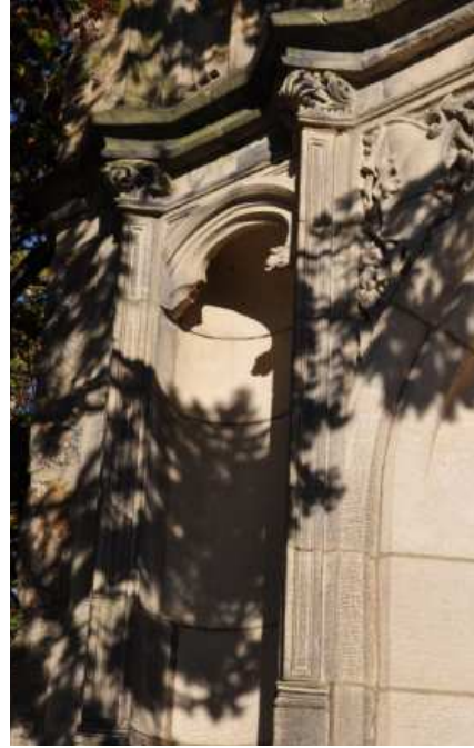
Photo 6: Missing Stone at niche
