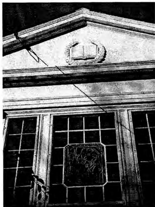
Figure 4: South gable end. Note carved pediment ornament and stained glass panel behind storm windows.
