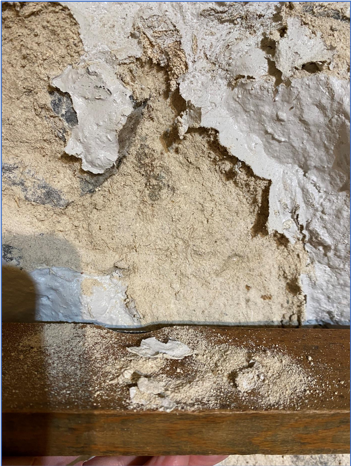
Fieldstone foundation wall, west. Mortar is crumbling and during rainy weather it is thoroughly wet (muddy).
