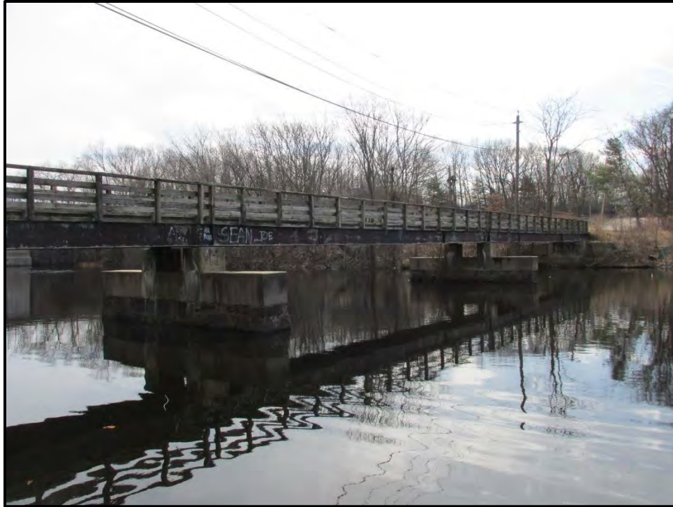
Photo 1: View of the existing bridge facing southeast from the north (Newton) side of the Charles River.
