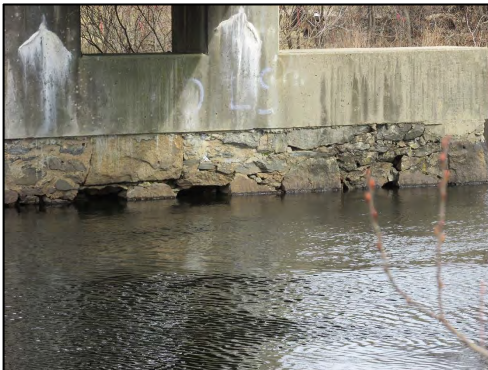
Photo 6: Evidence of fracturing and collapse along the water line in the stone masonry piers. Fracturing is visible in the concrete caps.
