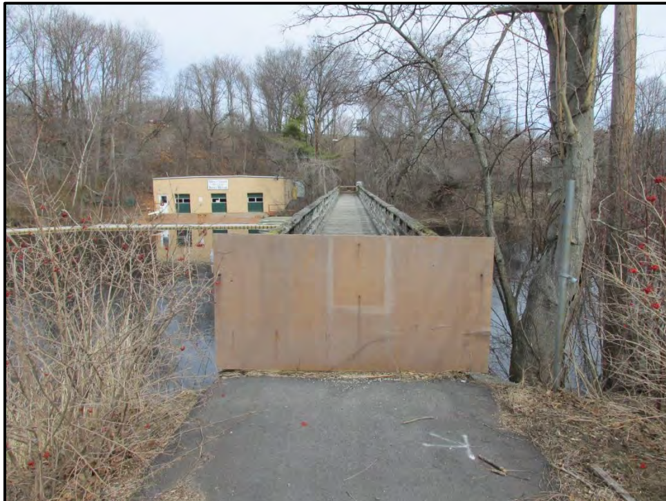
Photo 2: The south (Weston) end of the existing bridge has been closed to pedestrians using a sheet of plywood. The Lassell College Stoller Boathouse and docks are visible to the left of the bridge.
