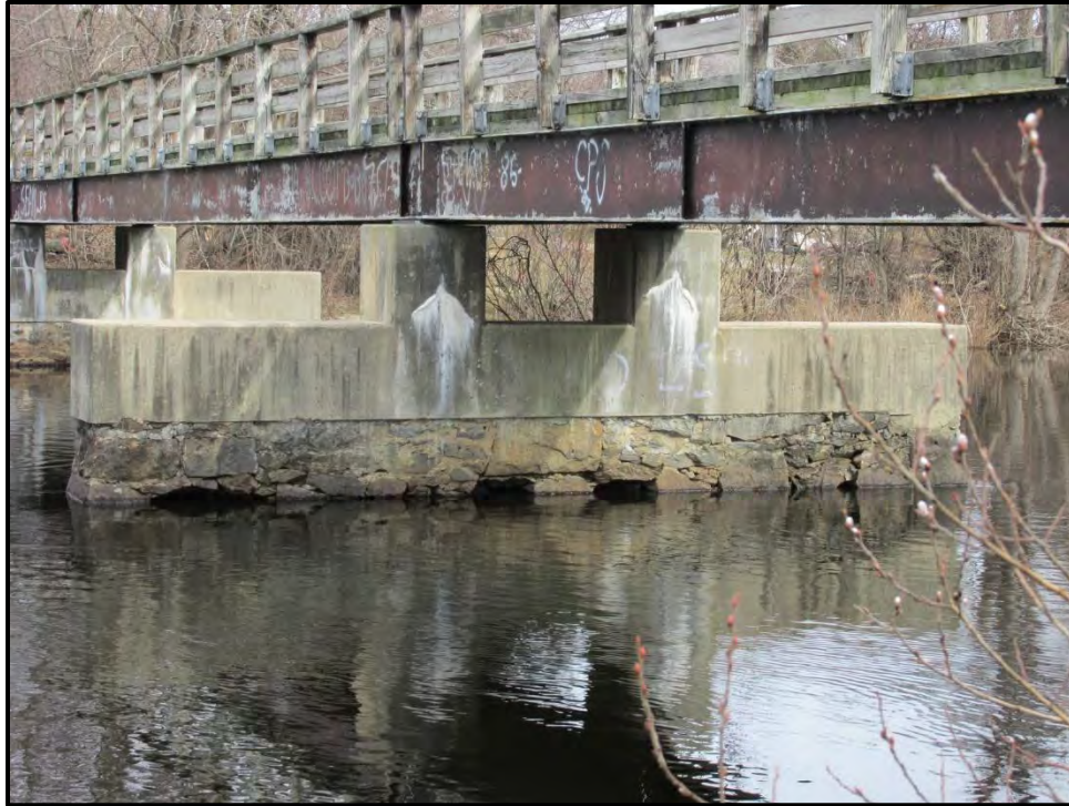
Photo 5: View of the existing stone masonry piers and concrete caps facing northeast from the south (Weston) side of the Charles River.
