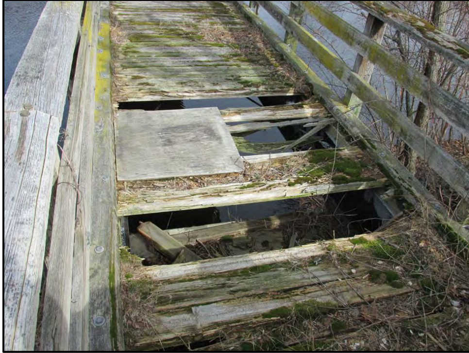
Photo 3: A collapsed portion of timber decking on the south (Weston) side of the bridge. The timber rails along both sides of the bridge also show significant signs of decay.
