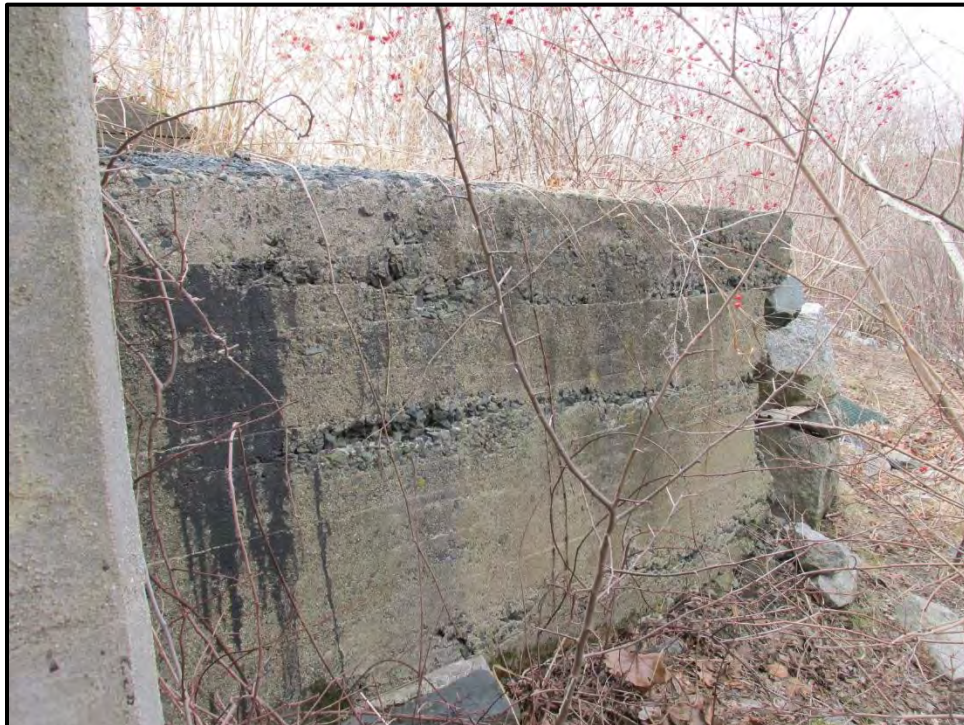
Photo 8: Evidence of fracturing and partial collapse in the north (Newton) abutment.
