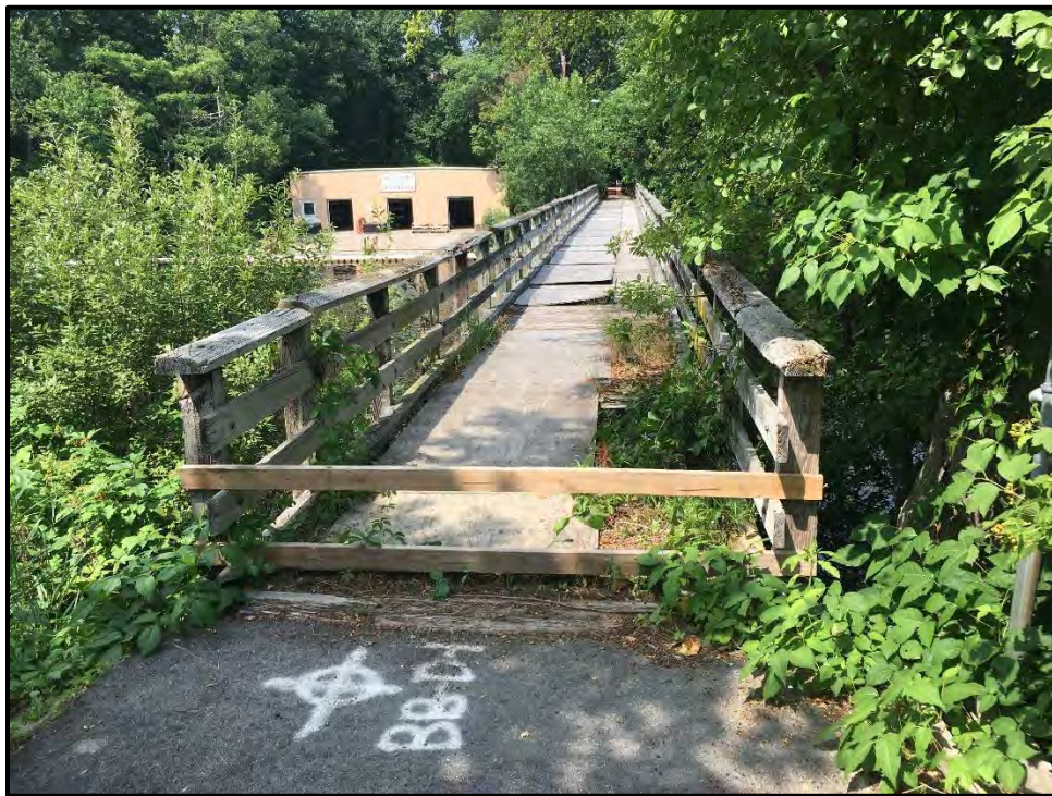
Photo 4: Though the bridge is closed to pedestrians, instances of trespassing are common and various methods of closure have been implemented (informally) by residents and local organizations. This photo shows multiple sheets of plywood laid over the collapsed portions of the timber deck to mitigate the safety hazard.
