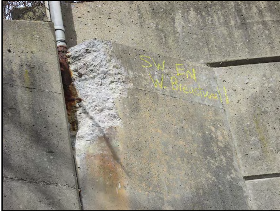
Photo 7: Fracturing in the southwest (Weston) breast wall.
