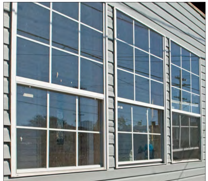
The 9-over-6 vinyl replacement windows have applied muntins, are mounted flush against the outside wall and lack the depth of traditional windows. They do not have trim or casings. They are not appropriate for historic buildings.
