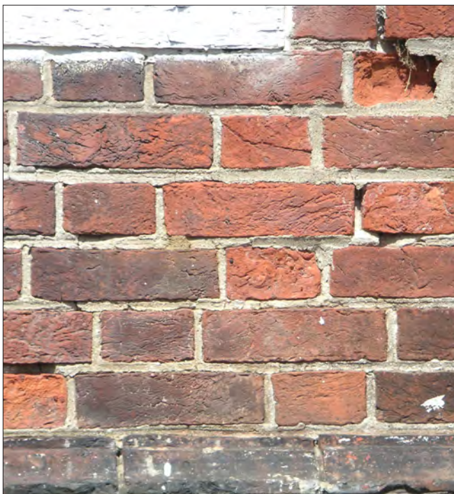
The repointing mortar in this wall is likely harder than the bricks, containing too much Portland cement. The surface of the upper brick has spalled, exposing the softer interior of the core. The mortar is also beginning to crack and pop out of the lower joints.
