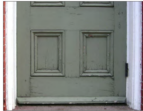
Wood checking and peeling paint is visible. Minor repair and maintenance can prolong the serviceable life of this door.
