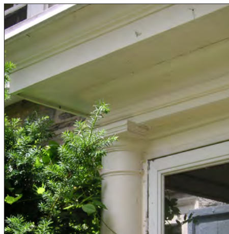
Porch enclosures that are attached to existing decorative porch elements such as this column can cause damage that is both difficult and costly to repair.
