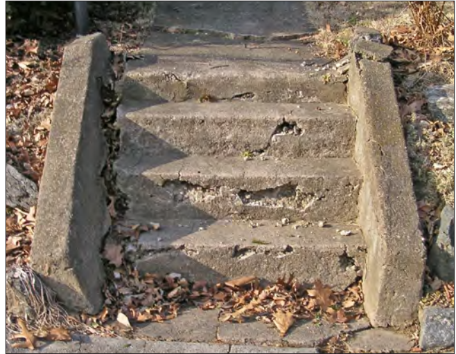
Without proper upkeep, tripping hazards can develop at steps and walkways. There are significant cracks and openings at these steps, exposing the reinforcing bars to stormwater and de-icing salts. This can accelerate the rusting of the reinforcing and deterioration of the concrete.
