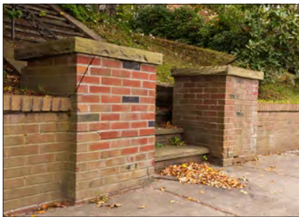
Similar to building walls, landscape walls and fences require regular maintenance, particularly at retaining walls. There is significant cracking at both of the piers that might indicate a structural problem.
