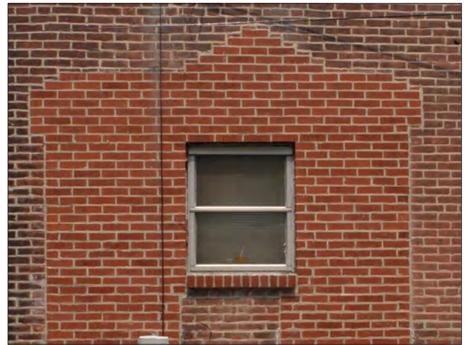
The brick infill area is clearly visible. The infill area uses bricks of a different size and color than the historic bricks and is outlined by a thicker mortar joint rather than being "keyed" into the adjacent brickwork. The bricks and mortar used in the infill areas should be the same size, color, texture, appearance, profile and hardness as the adjacent historic bricks. The repair should also be "toothed" into the adjacent brick to appear continuous with the wall surface.
