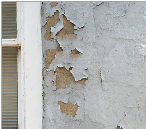
The peeling paint is likely incompatible with the stucco or caused by moisture. Loose and flaking paint should be removed and peeling cause determined before repainting.
