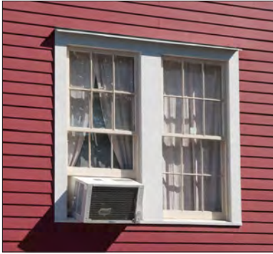
Installing window air-conditioning units in historic buildings is not encouraged, due to their appearance, likelihood of damaging windows and frames, and low efficiency.
