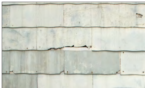
These asbestos shingles are cracked and worn. If replacement is considered, removal should be completed by a trained contractor.
