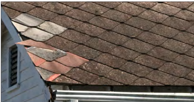
Asbestos roofing shingles came in various shapes, with diamond-shaped being the most common. This asbestos roof has some non-asbestos replacement shingles of similar size and shape as the existing roofing.
