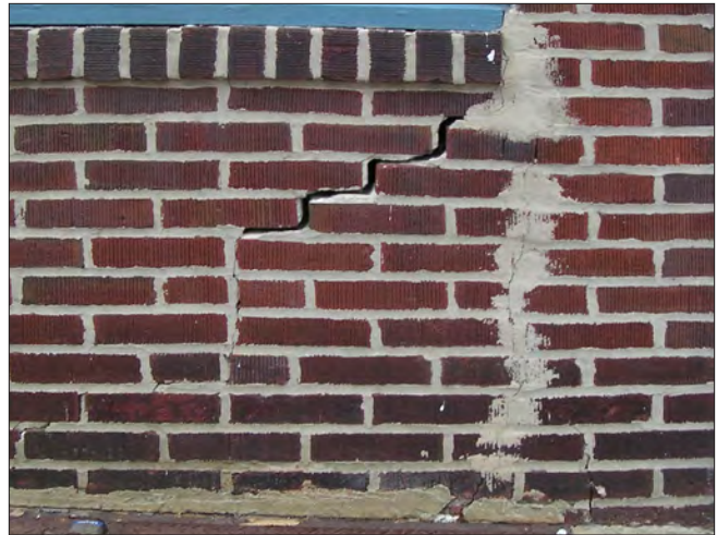
A previous vertical crack has been improperly repaired with hard grout smeared onto the wall surface. The second diagonal crack suggests a settlement or movement problem, that warrants consultation with an architect or engineer.
