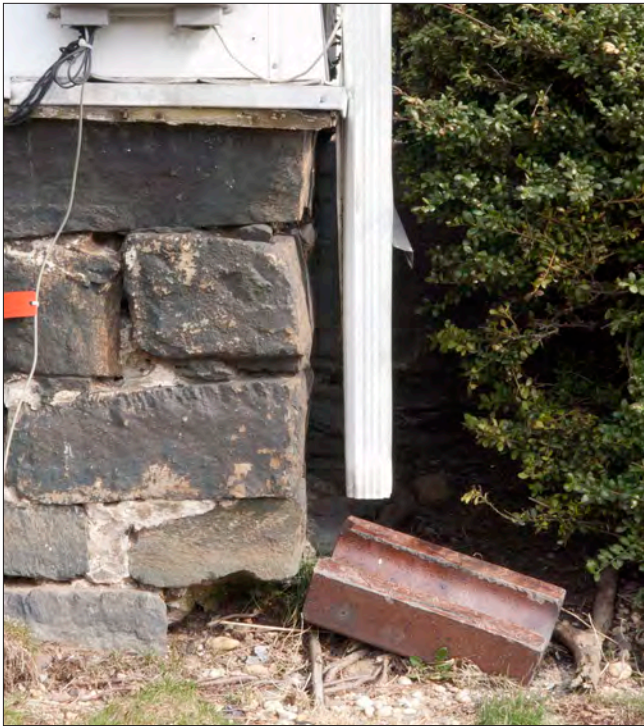
The storm water from the downspout has deteriorated the foundation's mortar and the bottom stone has been dislodged. It is recommended that water from the downspout be directed at least 3 feet away from the foundation and that the shrubs be trimmed or relocated away from the building.
