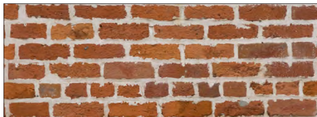
This photograph illustrates an inappropriate repointing of historic brick. A saw was used to cut-out the joints during repointing, extending the vertical joints. In addition, both the vertical and horizontal joints have been widened.
