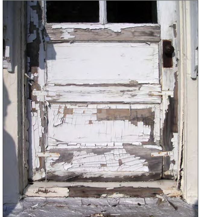
The paint on this door has alligatored, and severe cracking is visible. Removal of paint down to bare wood and proper door repair are recommended prior to repainting.
