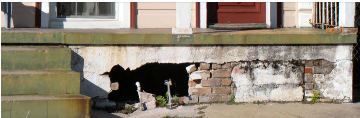
The stucco has not been maintained and the bricks under the porch post are falling out of position. The dislodged bricks can lead to structural problems in the porch if not repaired.
