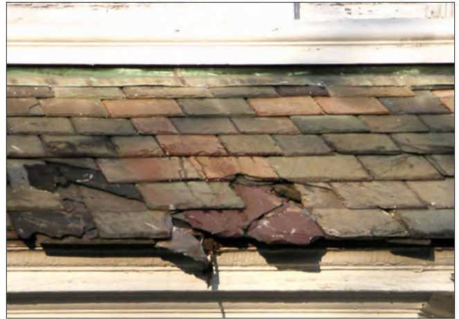
Slates are cracked, dislodged and missing. Some of the surfaces are delaminating. Approximately 25 to 30 percent of the slates on this roof are either missing or damaged. Given the pervasiveness of the problems, considering roof replacement would be appropriate.
