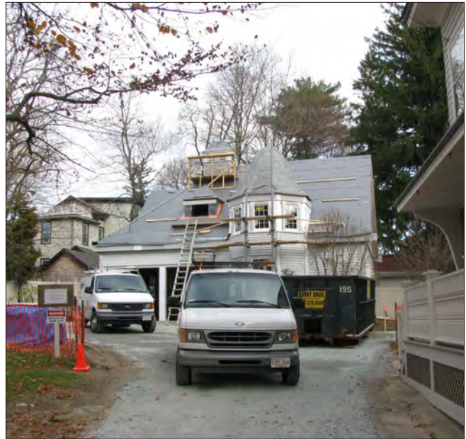
This carriage house at 43 Fairmount Avenue is being adapted for reuse as an office. The work is being funded in part through state and federal tax credits.
