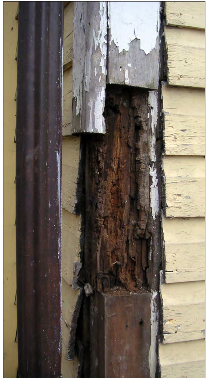
The vertical wood corner boards were removed adjacent to the downspout exposing the structural wood post. Additional exploration revealed that there was significant rot of the post that extended deep into the thickness of the wood, compromising the structural capacity. It is likely that a persistent leak at the juncture of the roof gutter and downspout made the situation much worse.
