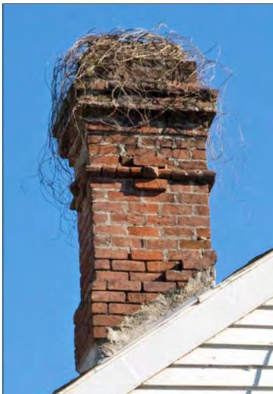
This chimney is leaning and has several visible open joints. Rebuilding to match existing detailing is recommended.
