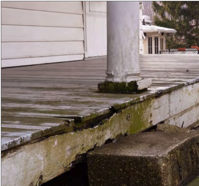
Porches, steps and other areas where the woodwork is laid horizontally or located close to the ground are often first to deteriorate. Ongoing exposure to moisture can lead to rot of the column bases, porch deck and apron.
