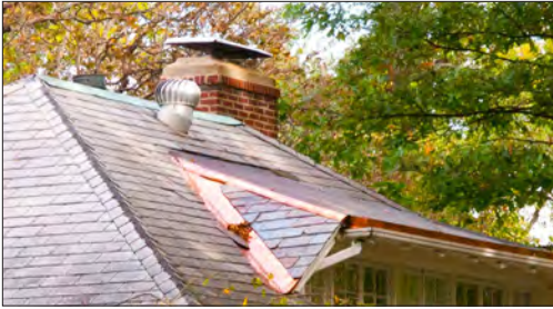
Flashing is commonly found at chimneys, dormers and intersections of roof forms.
