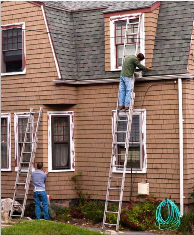
General maintenance, including repainting of woodwork, is essential for preserving original building fabric and unique architectural elements and details.
