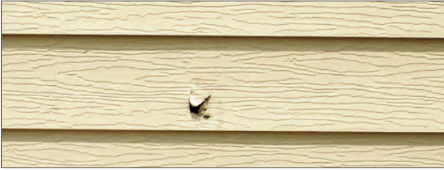
Replacement of this aluminum siding is the best way to repair this puncture. A wood-grained texture is inappropriate.
