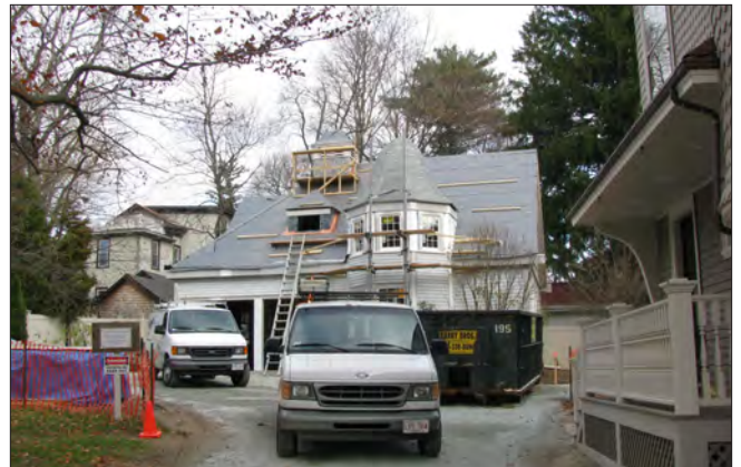
The work at this carriage house, at 43 Fairmount Avenue, is being funded in part through state and federal tax credits.
