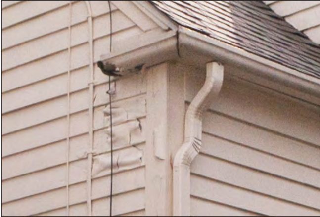
Paint problems at exterior woodwork are sometimes the first indication of an underlying moisture problem. The paint below the end of the gutter is peeling off the siding. Repairing the gutter and verifying that storm water is draining through the downspout is recommended prior to repainting.
