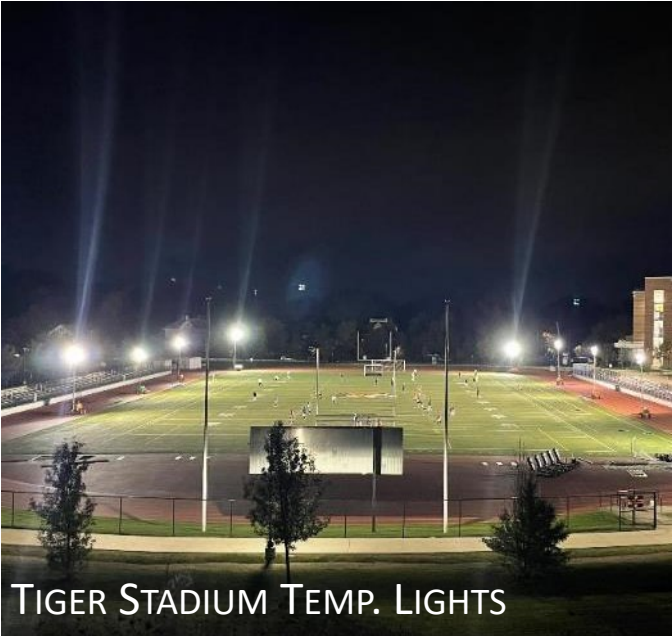
BRANDEIS RD. TEMP. LIGHTS
