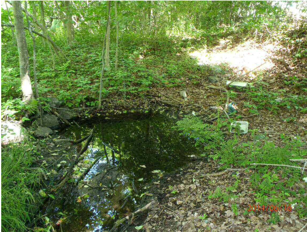
12-inch Submerged Outfall between #139 and #149 Harwich Road
