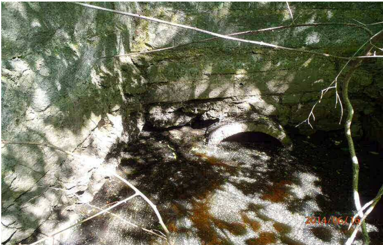
Close-up of Failing Headwall at Wayne Road Outfall
