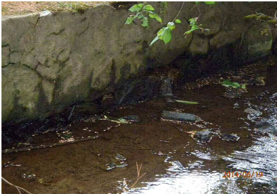
Underdrain Leaking into Hammond Brook
