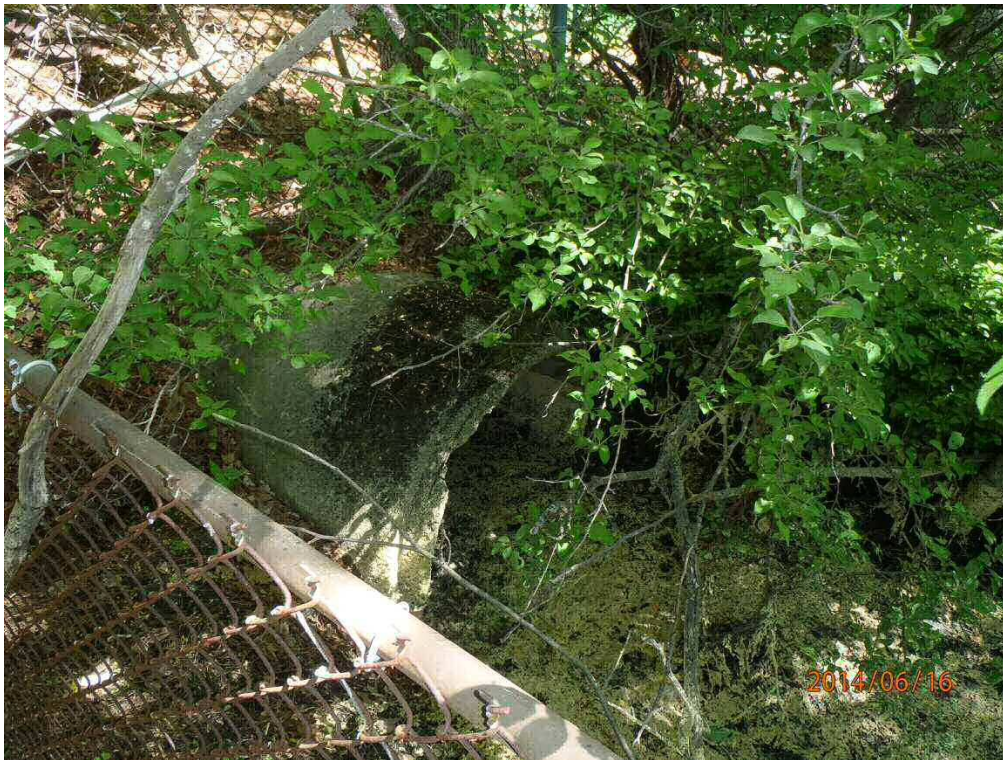
36" Outfall Off Harwich Road
