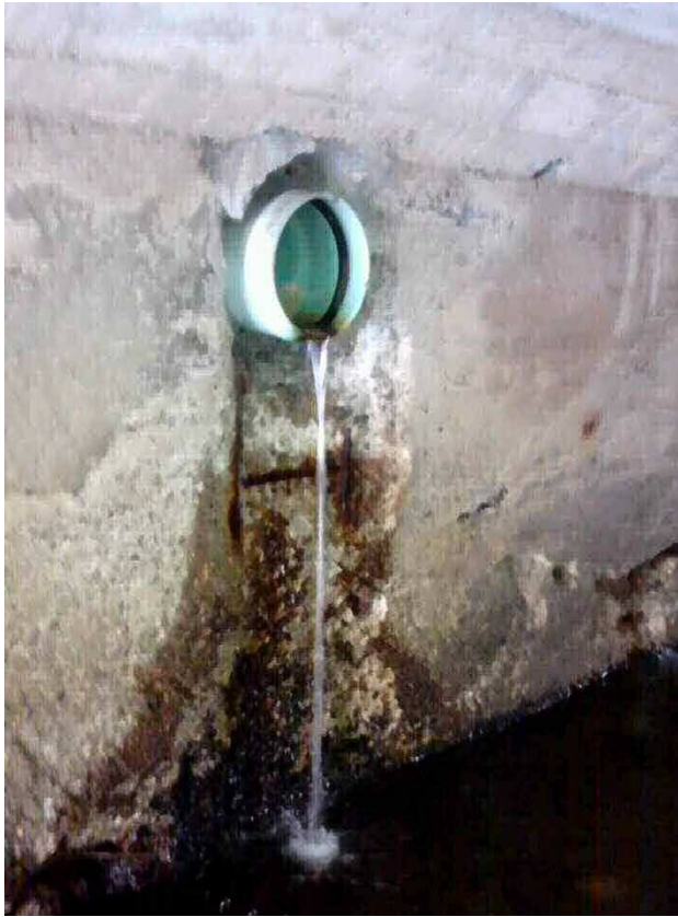
12" Outfall from Storm Drain on Dedham Street Discharging at Dedham Street Culvert
