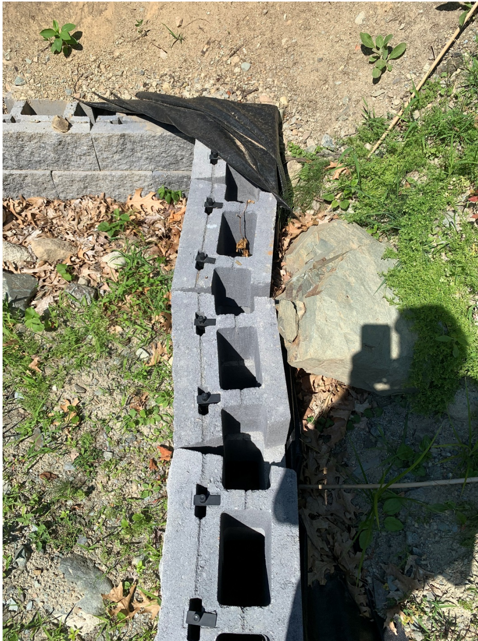
This large stone appears to have pushed out the two blocks
