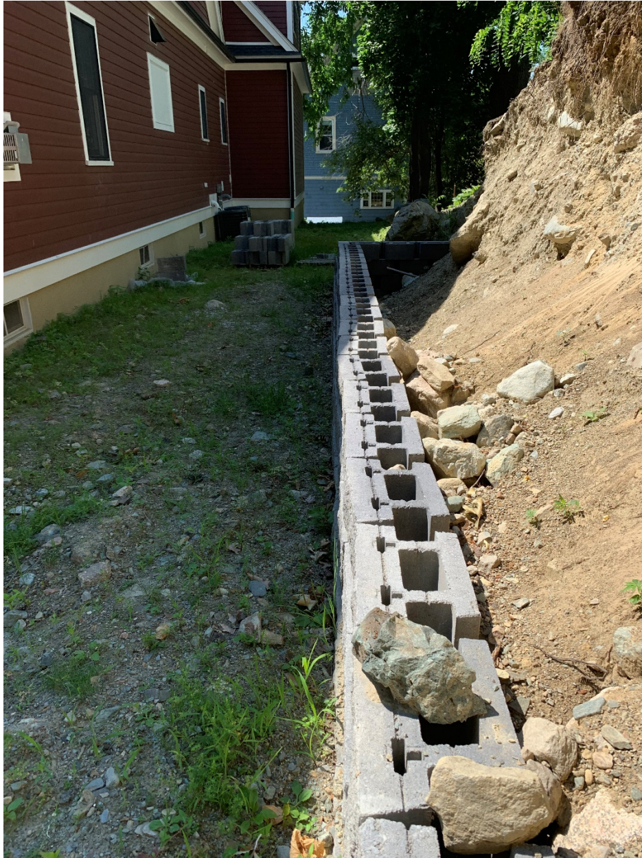
Multiple stones appear to have fallen and pushed out a couple blocks.
