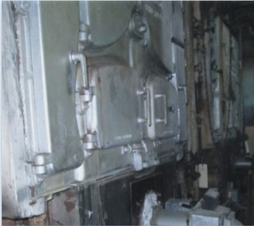
71-year-old oil-fired boilers at the Peirce School
