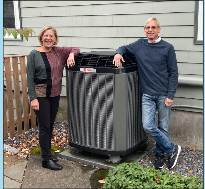
Karen and Jon Slote with the outdoor unit of their heat pump.
