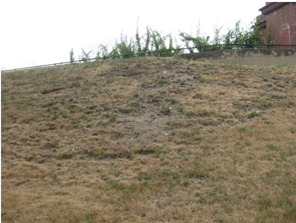
Waypoint 9: soil erosion on hill
