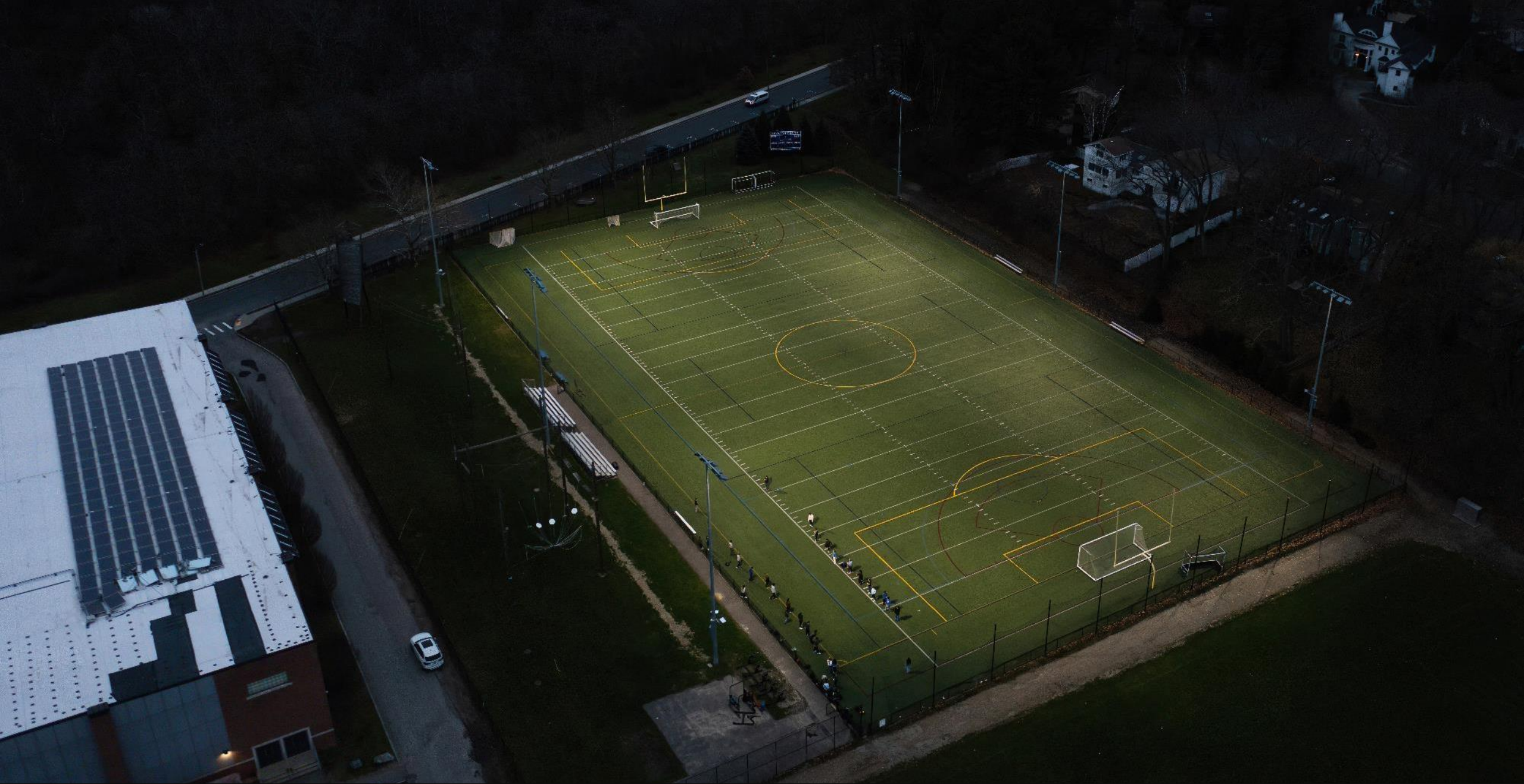
NEWTON SOUTH HIGH SCHOOL BRANDEIS RD FIELD SPORTS LIGHTING
